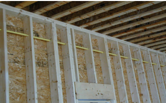
CSST installed through wall framing
